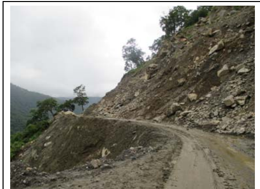
Sample of Road Slope Failure
