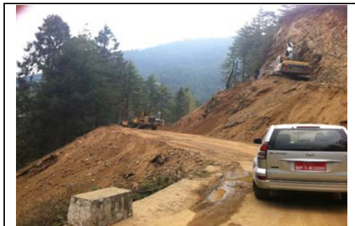
Aspect of Road Construction & Slope Failure
