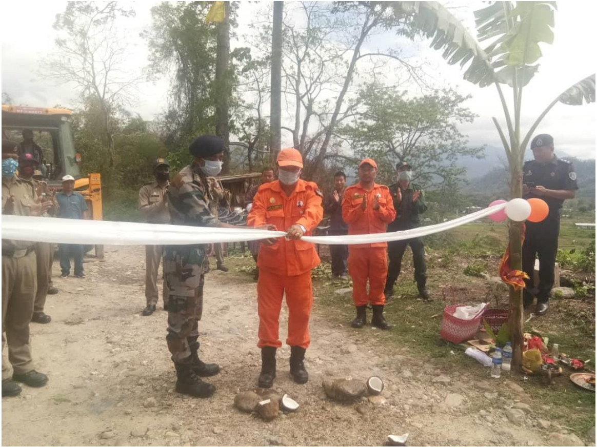
Ground breaking ceremony for FC works from Jomotshangkha side on 26 th April 2020 graced by Dasho Dungpa, Jomotshangkha Dungkha.
